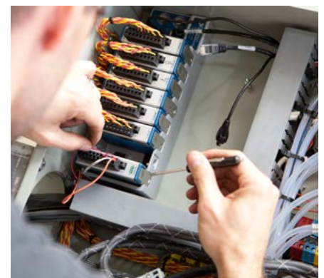
CompactDAQ in an industrial enclosure as part of engine test cell
