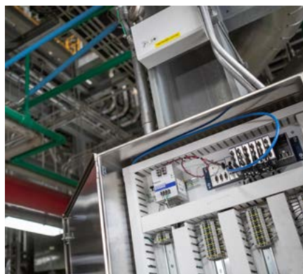
CompactRIO in an industrial enclosure installed in a power plant
